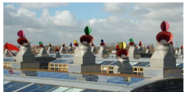
Figure 16. BedZED featuring passive ventilation chimneys, UK
