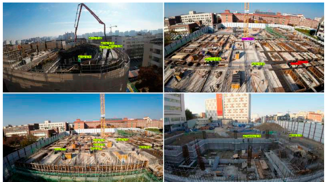
Figure 7. The visualization results of Liang et al.'s proposed automated detection method for helmeted workers using UAVs on construction sites [111].
