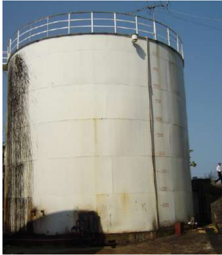
Fig. 1. A view of the liquid fuel storage tank.
